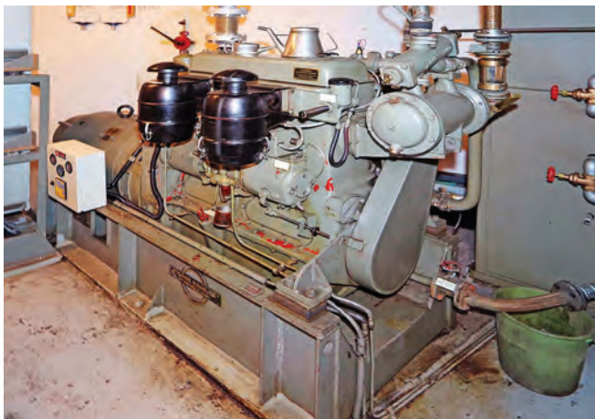
The 90HP generator within the Berliner Tor bunker
